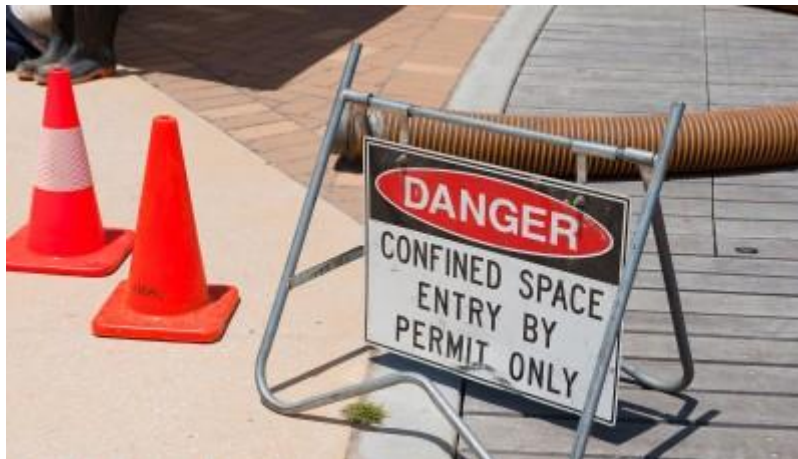
Figure 7 – Confined Space signage example
