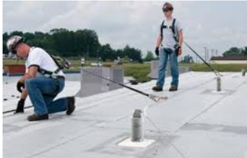
Figure 57 – Fixed static line on roof
